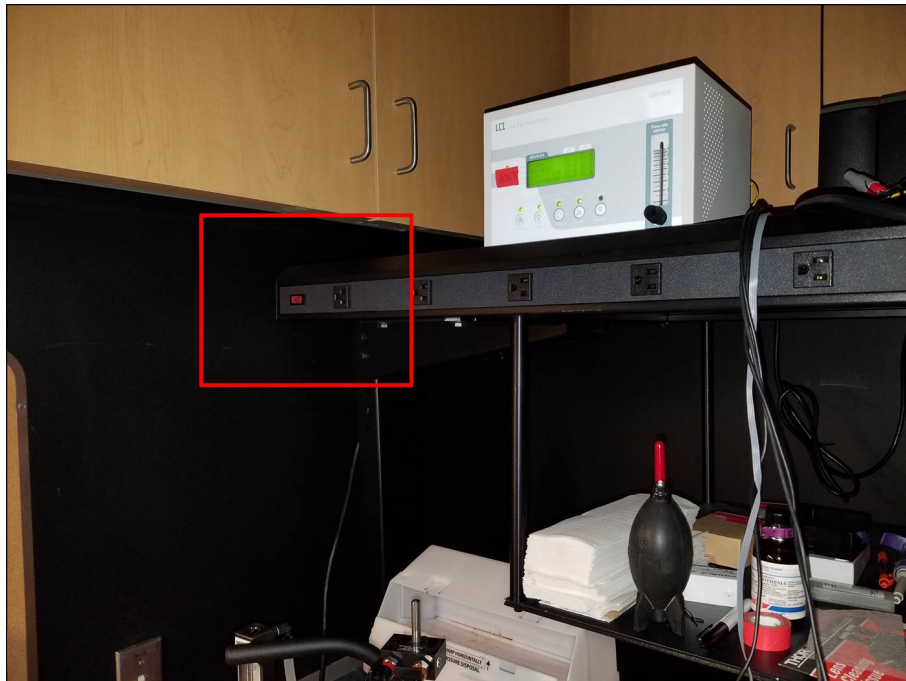
Figure 3: Power Strip for Components
